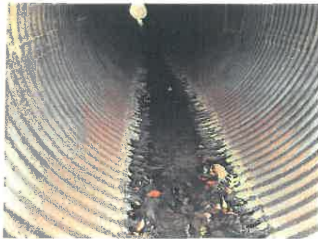
Rusting Out CMP Invert
