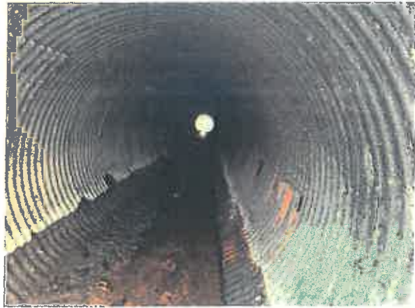
Rusted Out 60” CMP Invert
